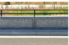
Example Barrier with Metal Railing that could be Used Next to Five Mile Creek.
